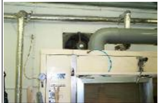
Afzuigventilator in de wand
